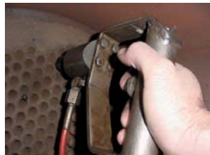
Instead of plugging the tubes we went in with sleeves that were roughly 7 ft. long and installed the sleeves in the ID of the tubes. The sleeves extended past the area where the stress cracking or excessive wall loss was located.
