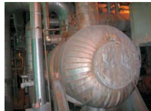
APS was able to extract a tube sample using their proprietary and patented advanced plasma arc tube cutter (P.A.T.C.), APS's plasma arc tube cutter enables them to cut heavy wall tubes at any length up to the tangent point of the U-bend in order to facilitate tube sample removal.
